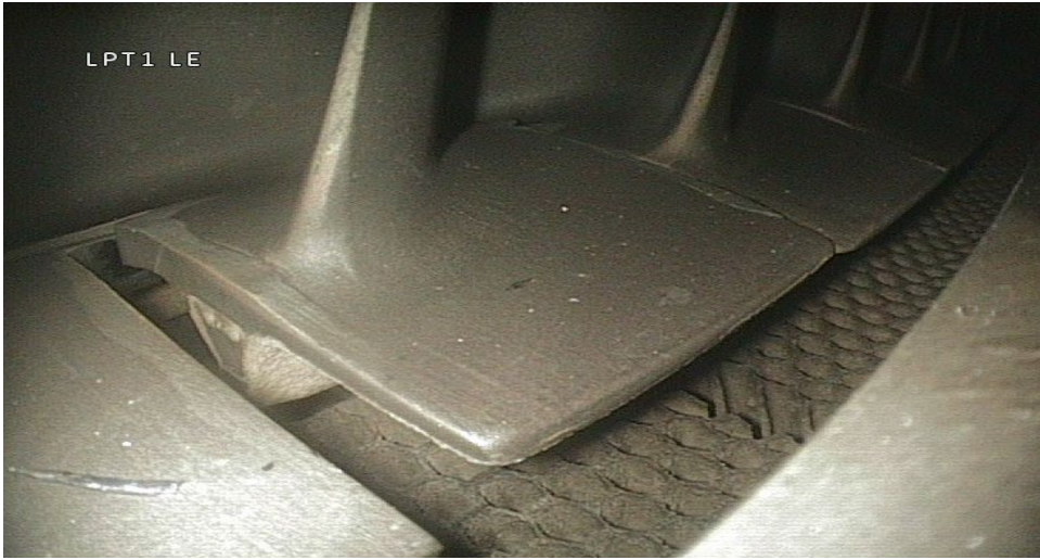
LPT 1 BLADES OBSERVED WITH GAP IN THE TIP SHROUD INTERLOCK. ACCEPTABLE AS PER AMM 72-00-00-200-808-F00.12.G.(2).(h).1.(a) THAT INTERLOCK FACES SHOW NO SIGN OF WEAR. SEE APPENDIX N FOR CLARIFICATION.
