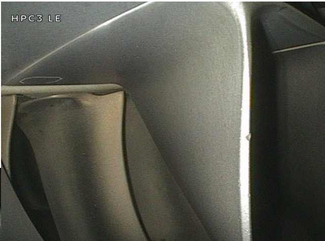
STAGE 3 HPC: SEVERAL HPC3 LE BLADES OBSERVED WITH MINOR DENTS TO LE IN LOWER 25%, DIM B & DIM A. ALL WITHIN AMM LIMITS. SEE DEFECTS PAGE FOR DETAILS. 1 OFF HPC3 BLADE OBSERVED WITH LE DENT IN AMM LIMITS. SHOP BLEND OBSERVED TO HPC3 TE ROOT RADIUS
